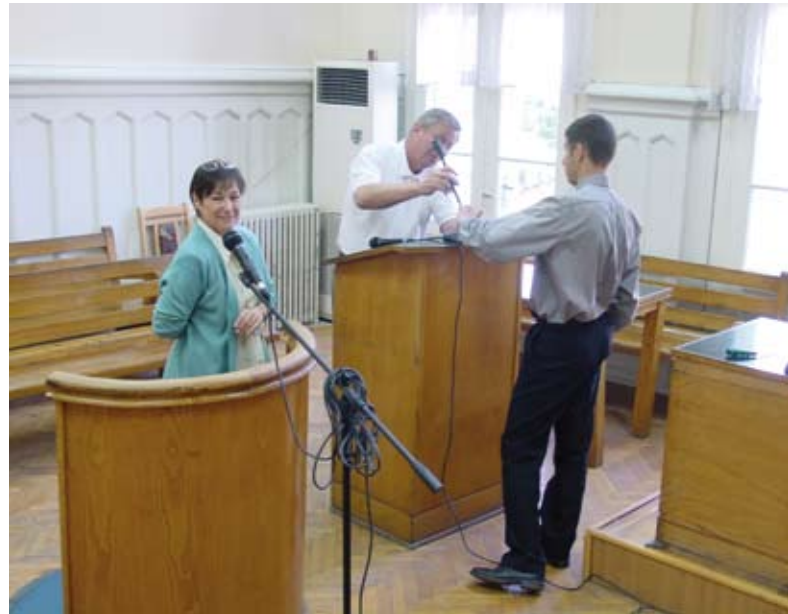
USAID Judicial Strengthening Initiative staff (center and right) assist the Shumen District Court with installing the Verbatim Audio Recording system in a courtroom.
